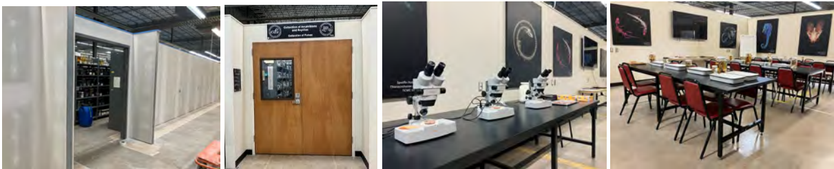
Figure 13 - Construction of new walls and security doors to define learning lab and wet collections workspace.
