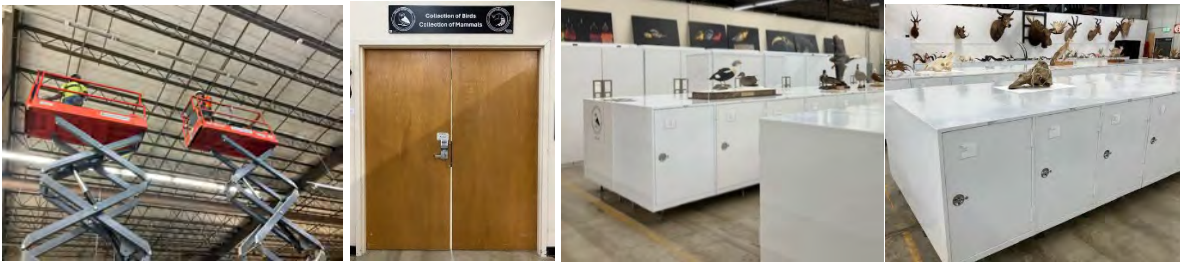
Figure 12 - Lowering of overhead lighting and installation of security doors leading to the bird and mammal range.
